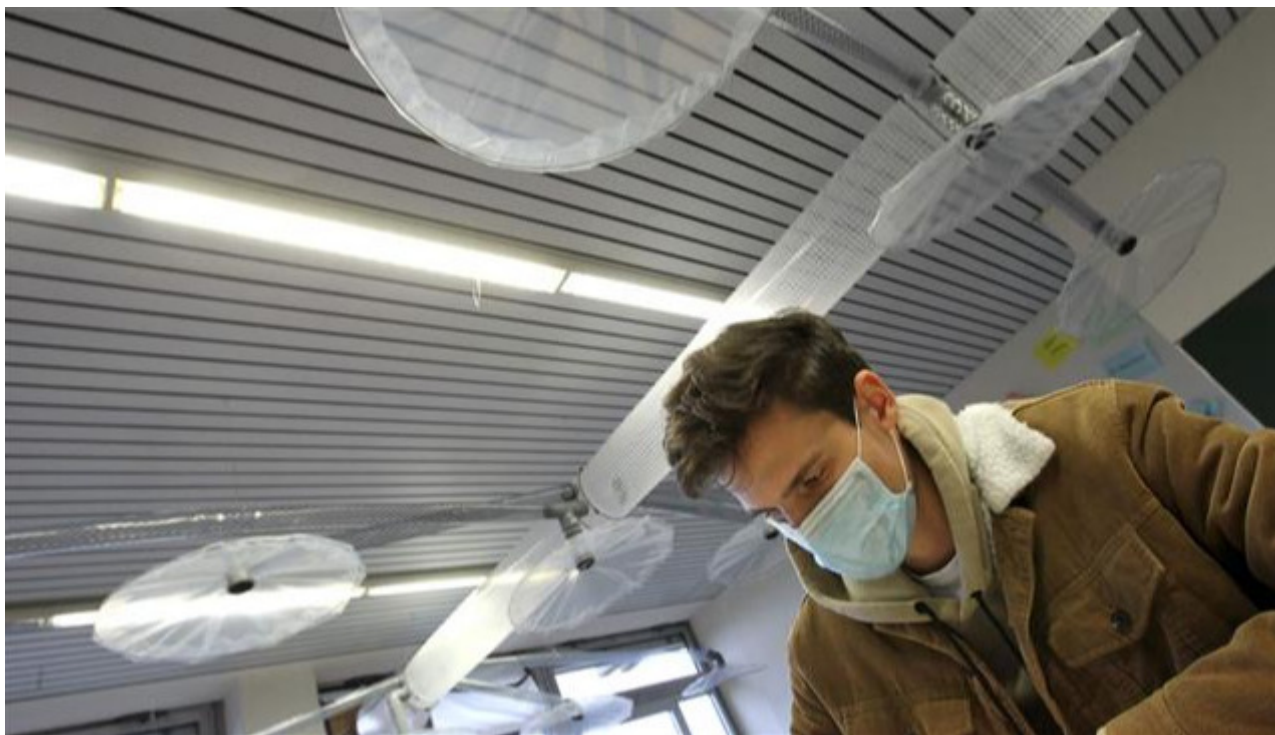
A ventilation system installed in a classroom is pictured at the IGS school in Mainz, western Germany. (Photo: AFP)
