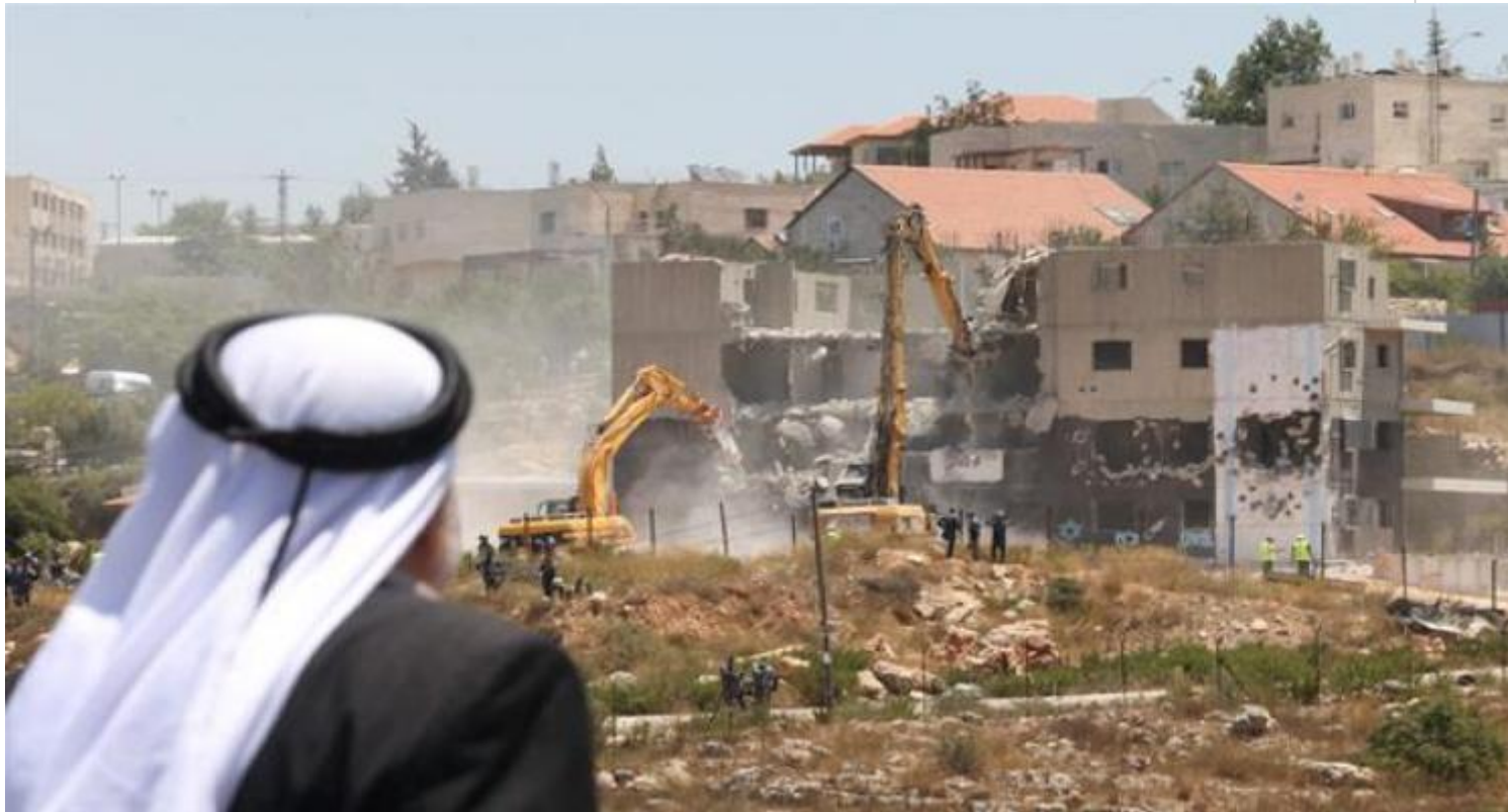
UN reports Israel demolishes 52 Palestinian structures
