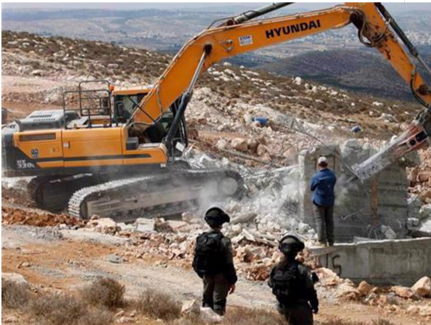
Israeli forces watch as a bulldozer demolishes a Palestinian house near the village of Beit Awa, west of the occupied West Bank town of al-Khalil (Hebron), on September 23, 2020. (Photo by
