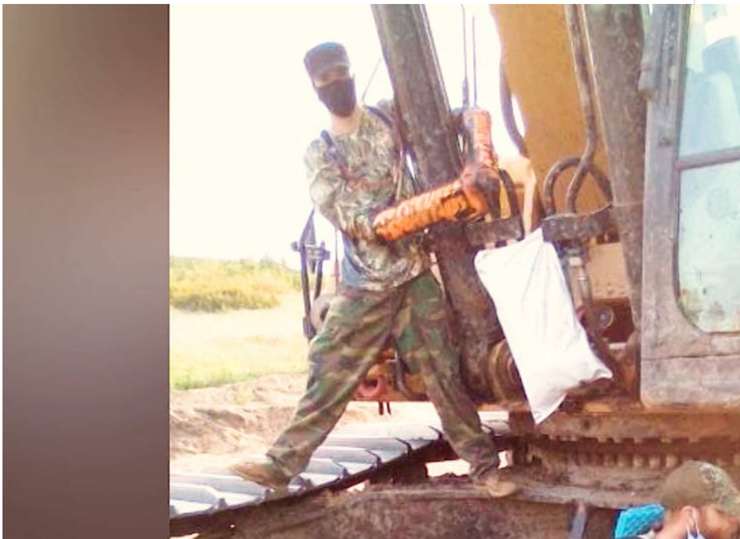
Water protectors take direct action to halt construction of Enbridge Line 3 Pipeline
