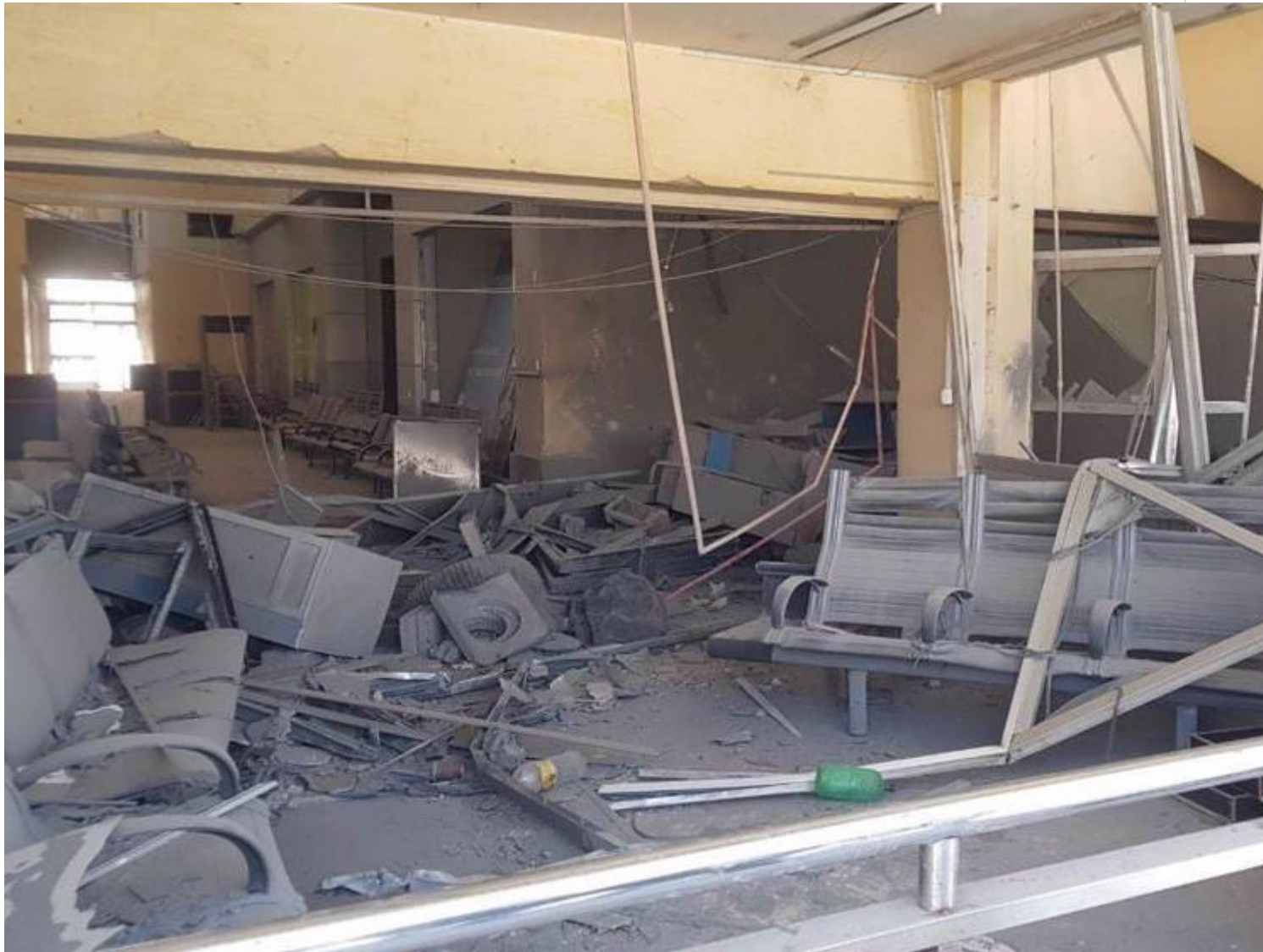
Damage is seen at the Damascus International Airport, Syria, after an Israeli airstrike, on June 12, 2022. (Photo by Syrian Arab News Agency)
