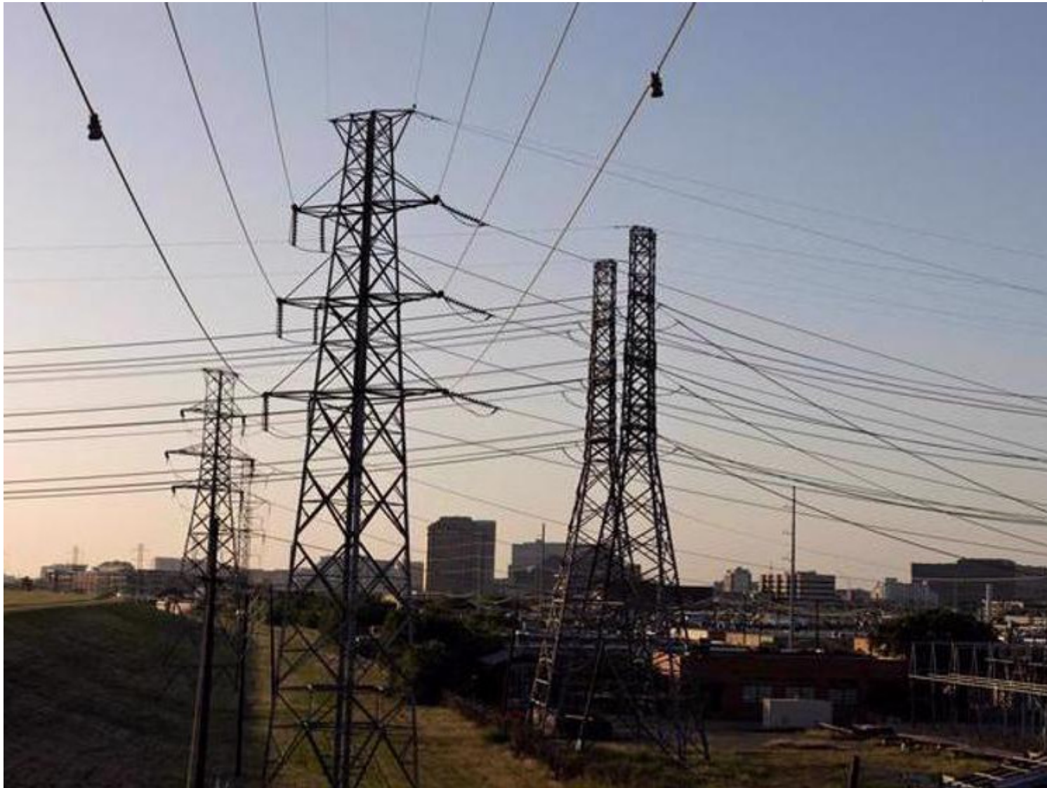
Power lines are seen during a heat wave with expected temperatures of 102 F (39 C) in Dallas, Texas, US, on June 12, 2022. (Reuters photo)
