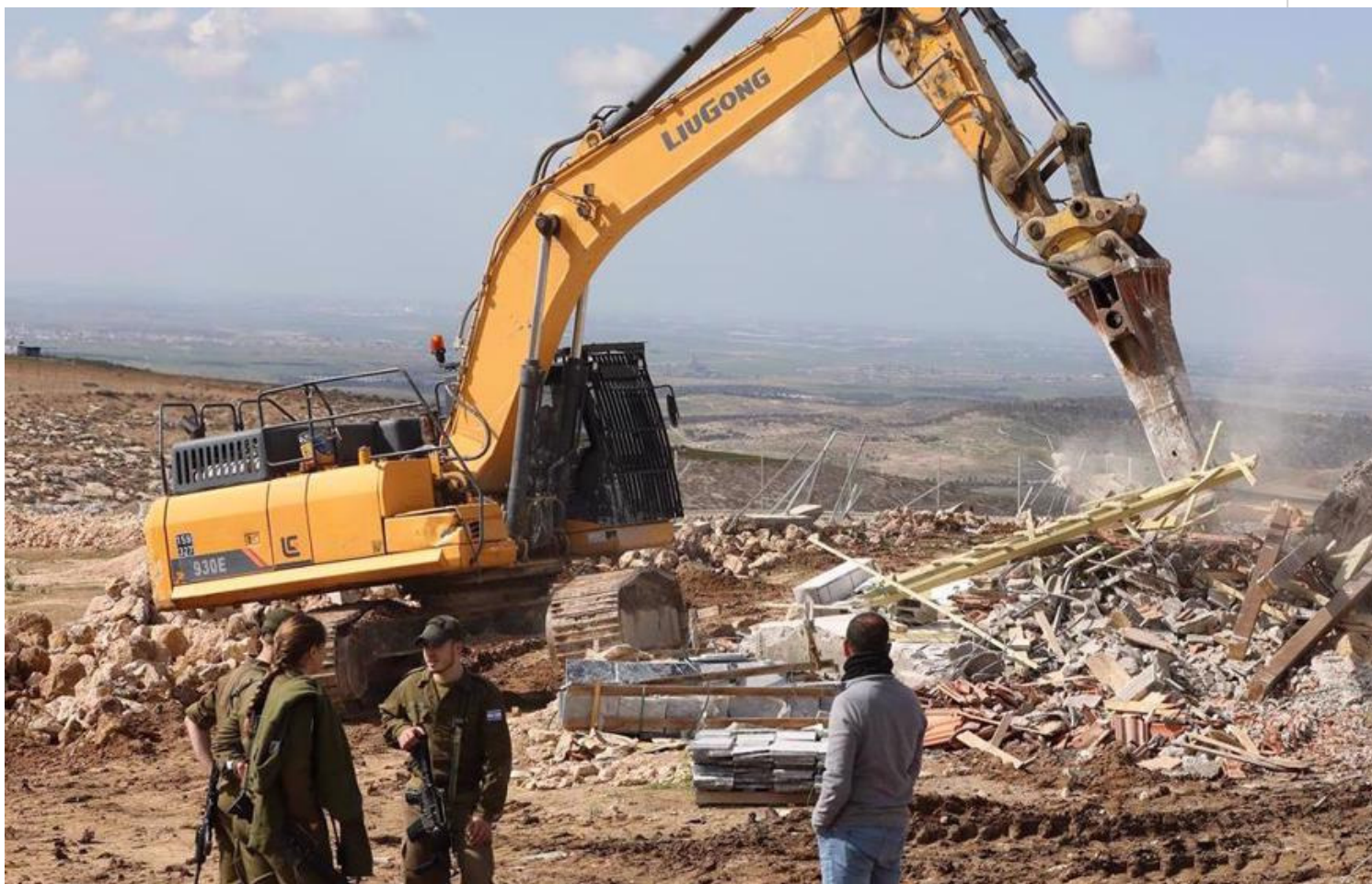
A bulldozer escorted by Israeli forces demolish a Palestinian-owned structure in an area of the occupied West Bank.
