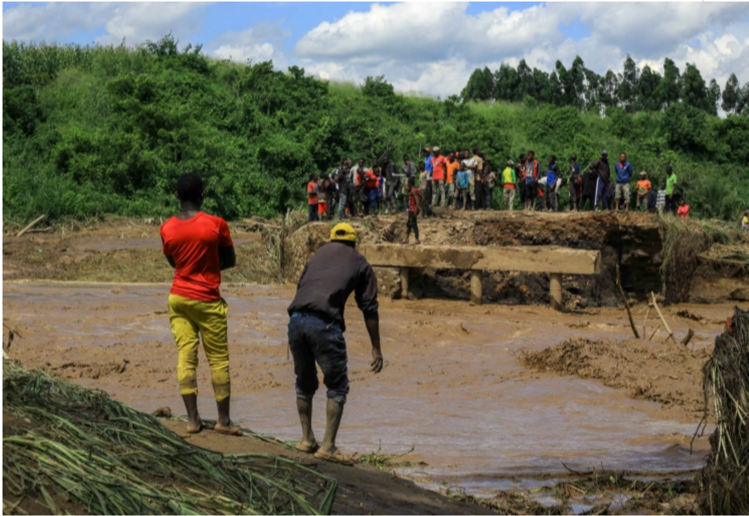
Residents gather near a washed-out bridge after flooding on the the River Hululu, which joins the Rver Lubiriha, near Beni, eastern Congo [File: Al-hadji Kudra Maliro/AP]
