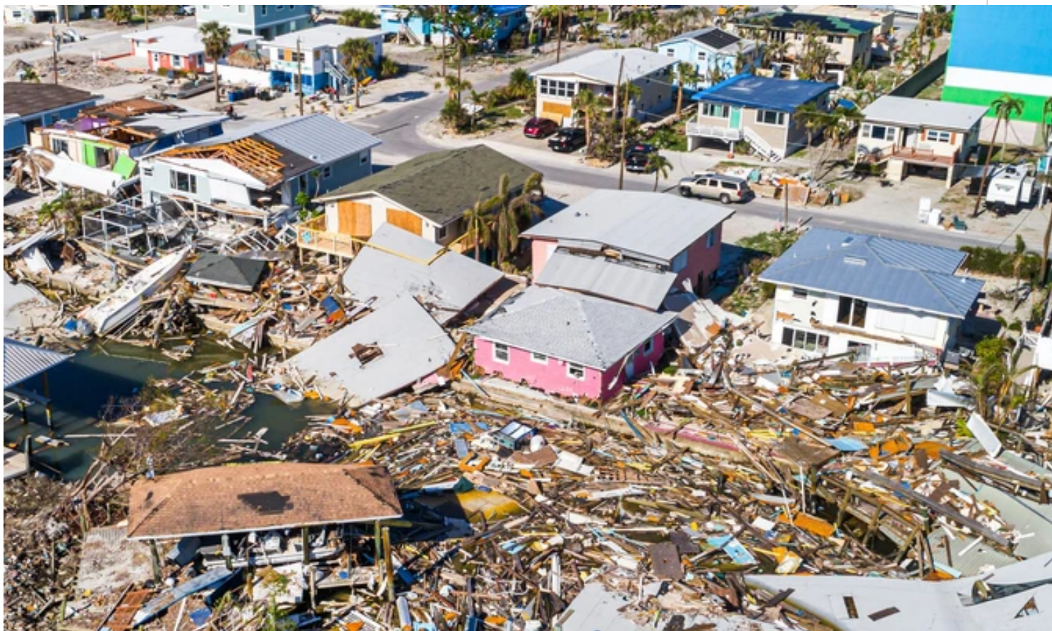
An aerial view of Ft. Myers Beach, Florida taken after Hurricane Ian shows homes, businesses, and property destroyed by the storm. (Photo: Jeffrey Greenberg/Universal Images Group via Getty Images)
