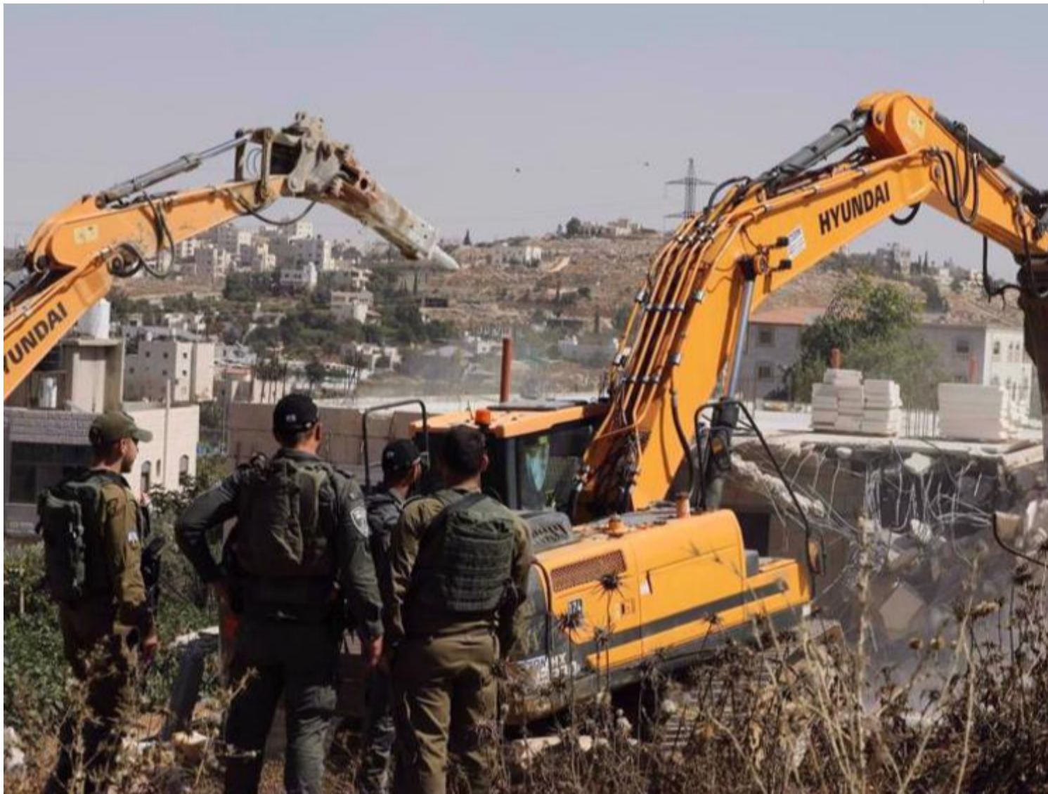
The undated photo shows Israeli forces demolishing a Palestinian house in an area of the
