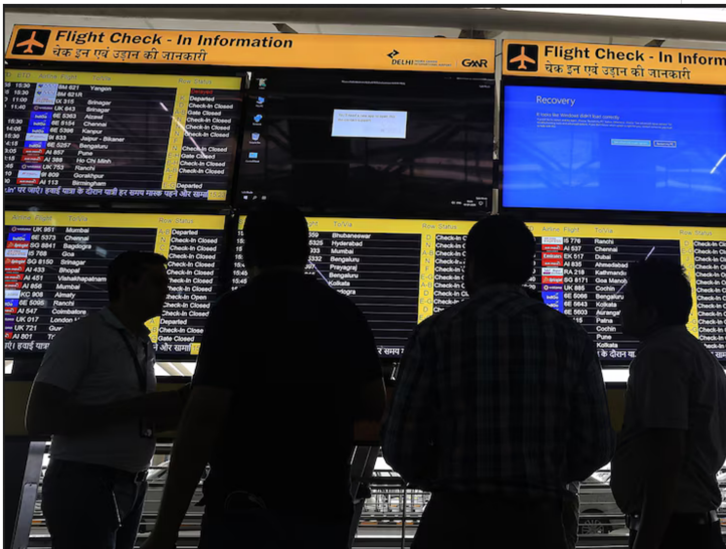
Indian workers try to repair a malfunctioning information screen at the Delhi International Airport
