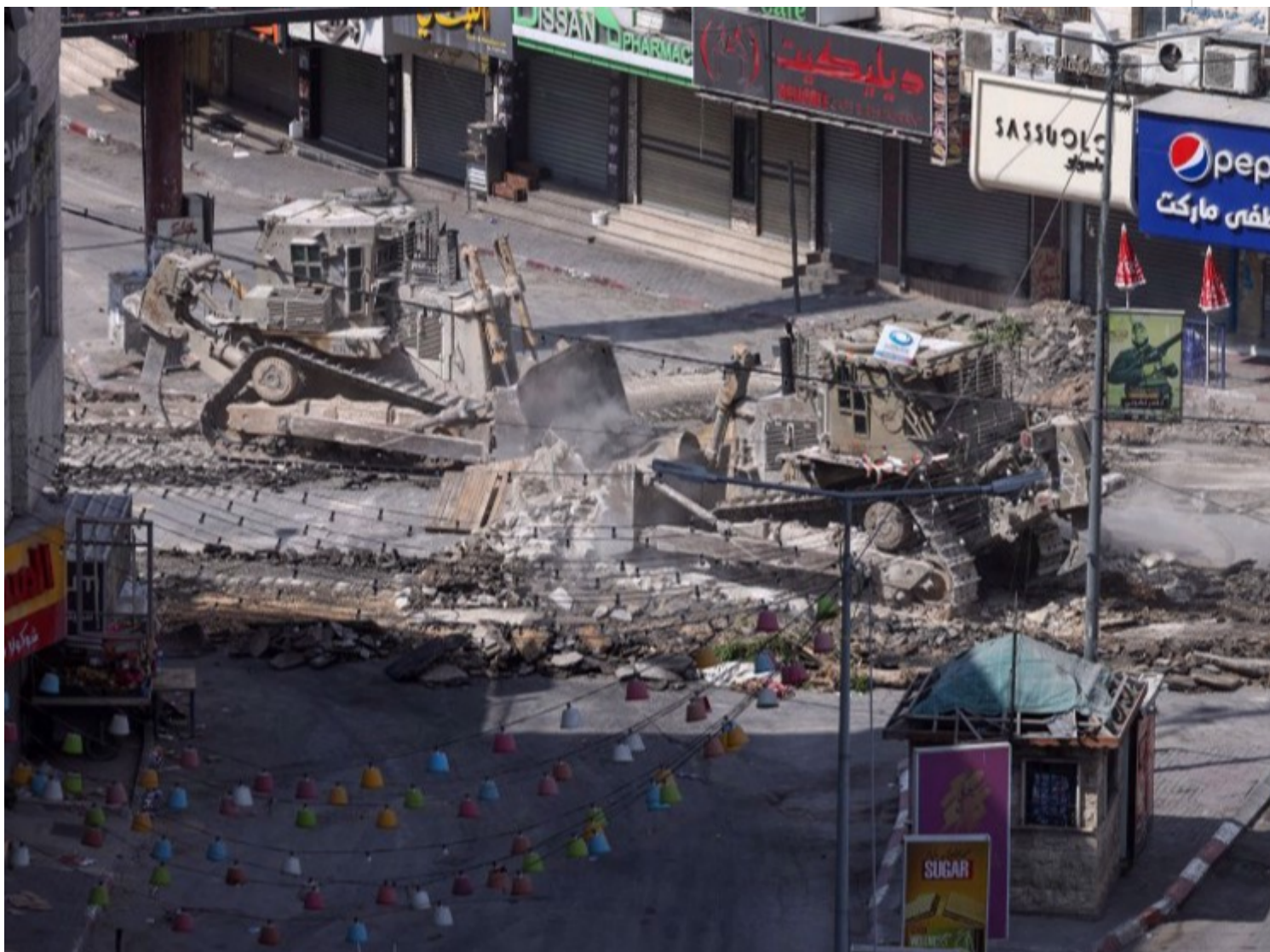
Israeli bulldozers tear up a street during an Israeli raid in the centre of Jenin in the occupied West Bank on September 2, 2024. (By AFP)
