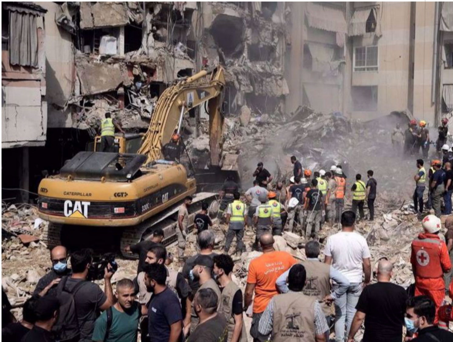
Site of an Israeli airstrike on a residential building in Beirut's southern suburbs on September
