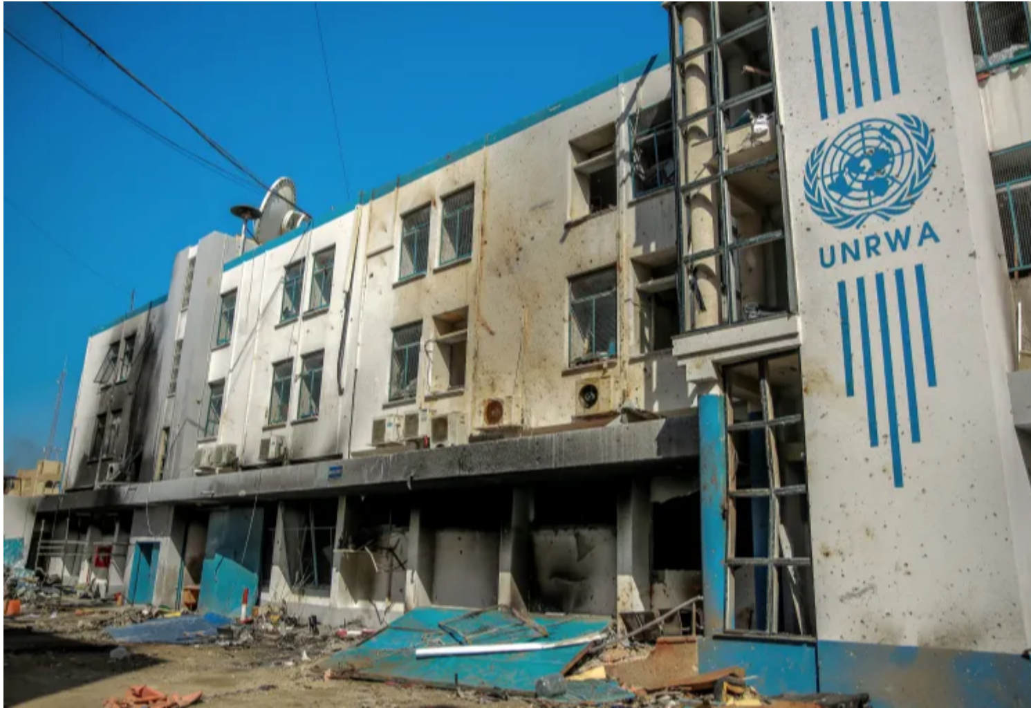
Photo shows the damaged Gaza City headquarters of the United Nations Relief and Works
