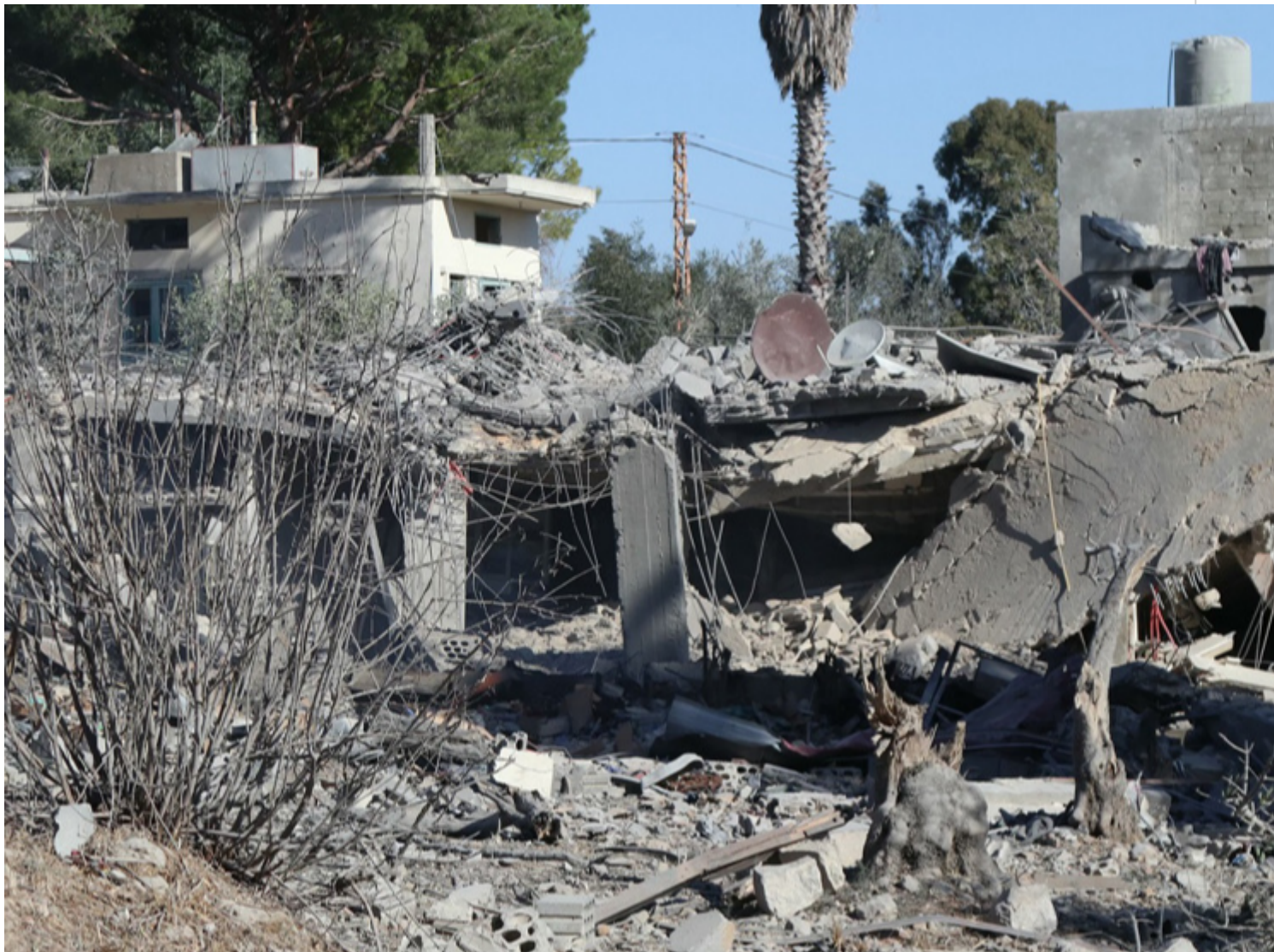
Photo shows the damage and destruction at the site of an overnight Israeli airstrike that targeted the southern Lebanese village of Marjayoun on October 27, 2024. (Photo by AFP)
