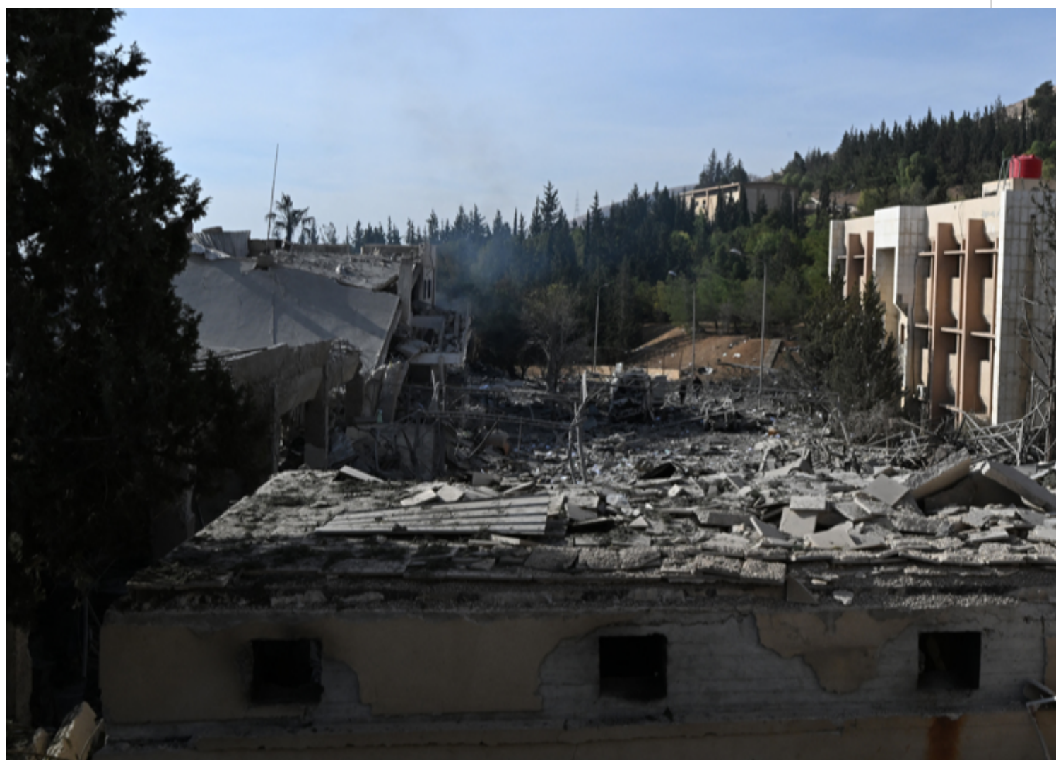
A general view shows the destruction at the Barzah scientific research center, north of the Syrian capital Damascus, on December 10, 2024, following an Israeli airstrike the previous day. (Photo by AFP)
