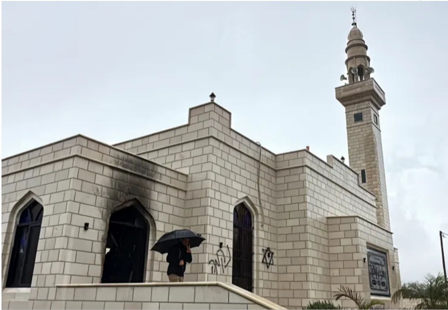
?The damaged mosque, burned by Israeli settlers, near Salfit in the Israeli-occupied West Bank December 20, 2024. RETUERS/Stringer
