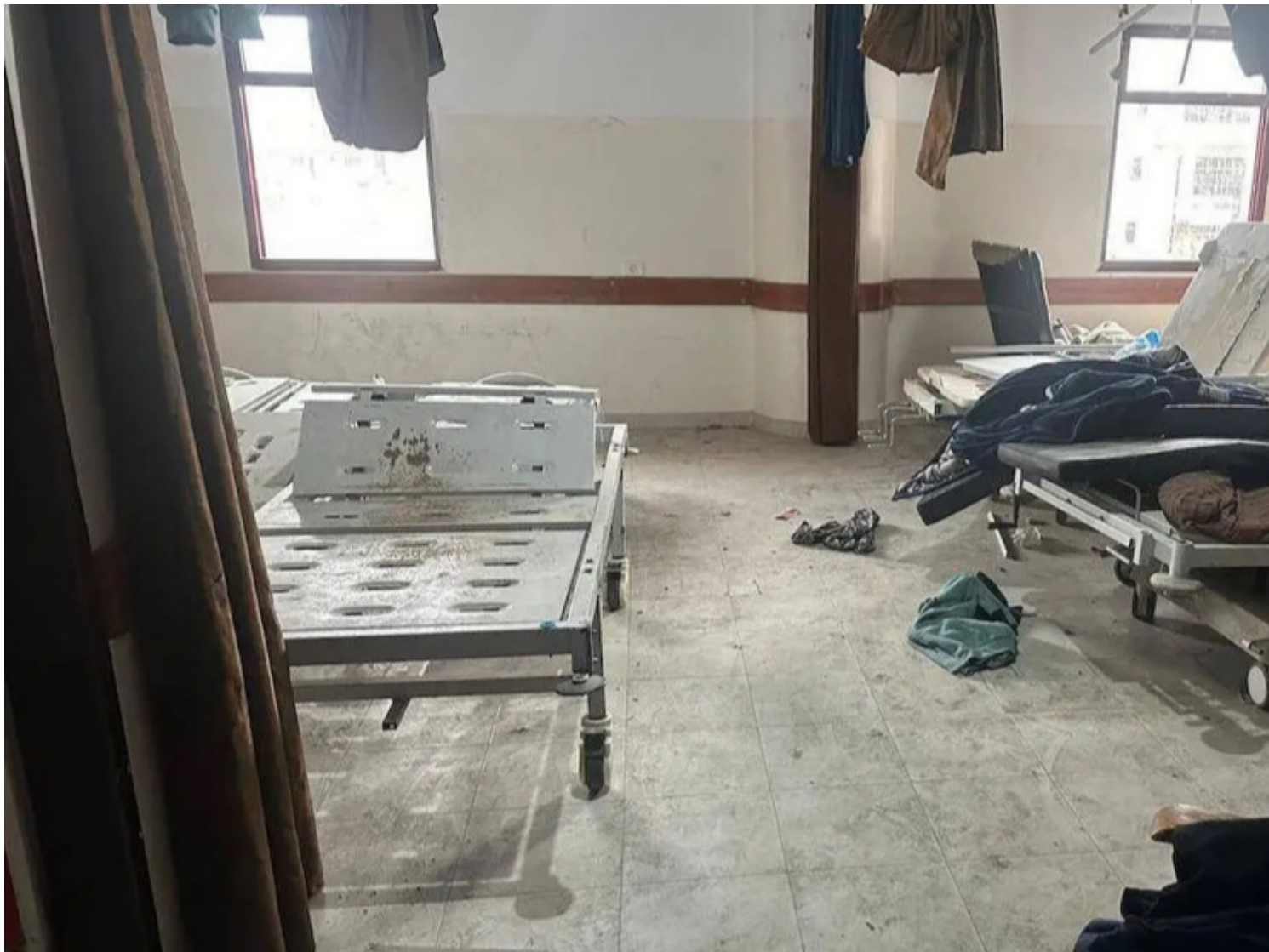
The Indonesian Hospital and many nearby buildings are damaged as a result of the Israeli
